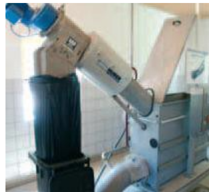
ASSEMBLED SYSTEM AT THE INSIDE OF THE BUILDING
