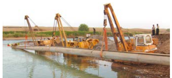
NATURAL GAS PIPELINE KHORMOR - ERBIL / N.IRAQ
