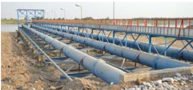
KUT - BADRAH - JUSSAN WATER TREATMENT and SUPPLY PROJECT / IRAQ
