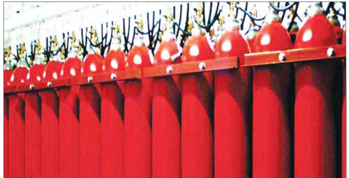
Co2 Fire Suppression Systems
