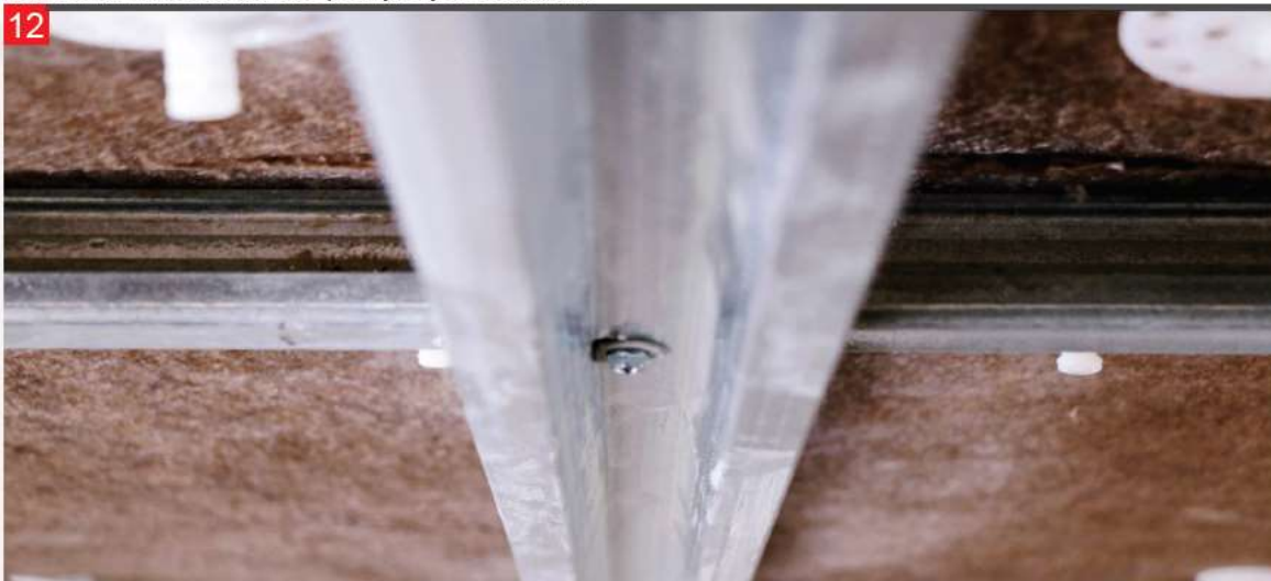
The M profiles that are used should be galvanized 20x80x3000 mm size and 0.50-0.55 mm thick. (The M profile dimensions and thickness may vary according to the static calculation).
