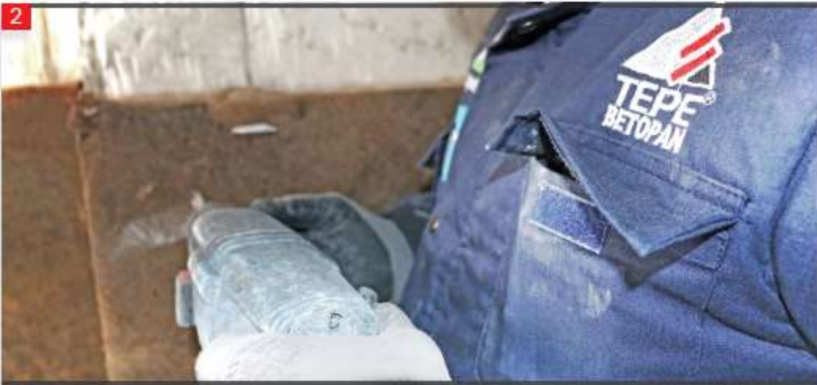
The necessary amount of stone wool is applied to the wall surface on the fixed L consoles.
