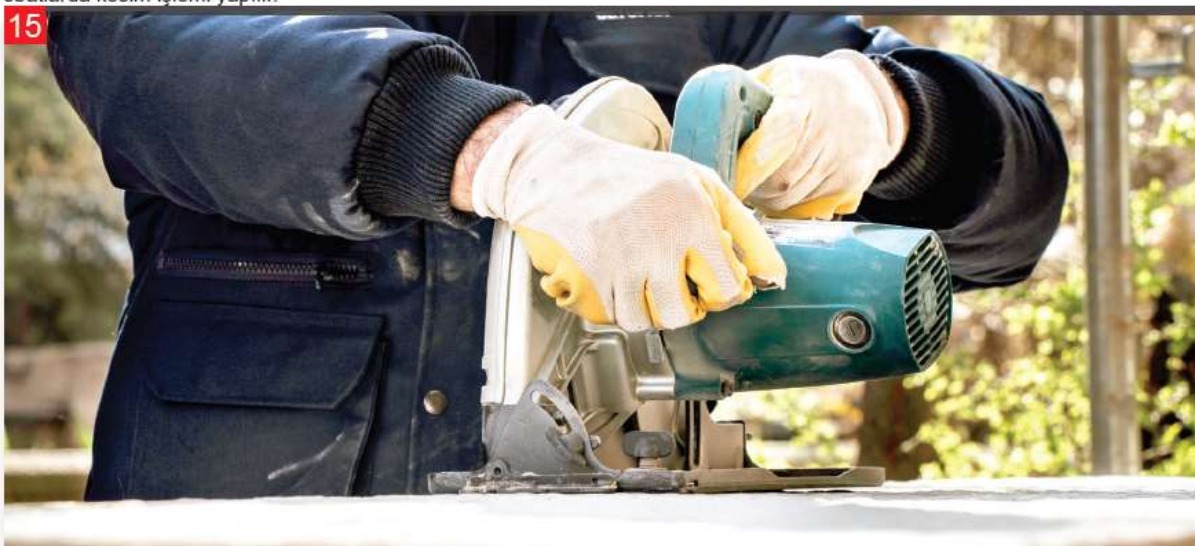
A diamond tip lateral cutter or diamond tip mobile cutter is used for the betopan group and circular saws especially produced for fibercement are used for the tepepan group.
