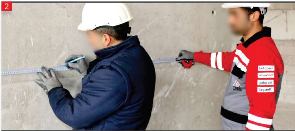
The position of the L consoles are determined and marked at 1 meter intervals. (May vary according to static calculation)
