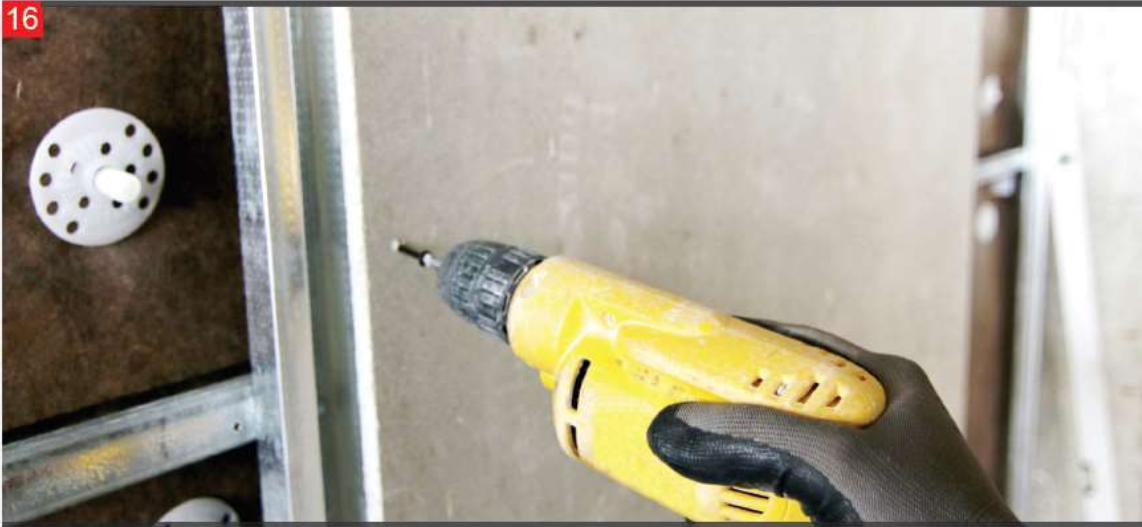
After the cutting process is completed the panels are mounted on the M profiles with rust proof screws.
