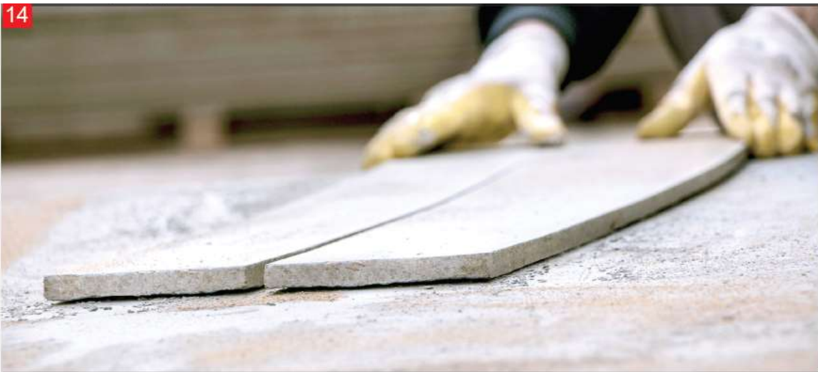
After the base construction stages are completed the panels are cut to the dimensions needed when starting the installation of the product.
