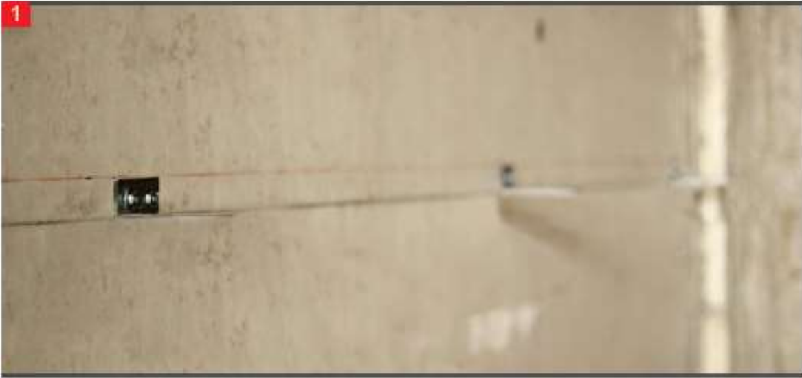
The curve of the application surface is determined and suitable L consoles to which the L profiles are to be connected are attached.
