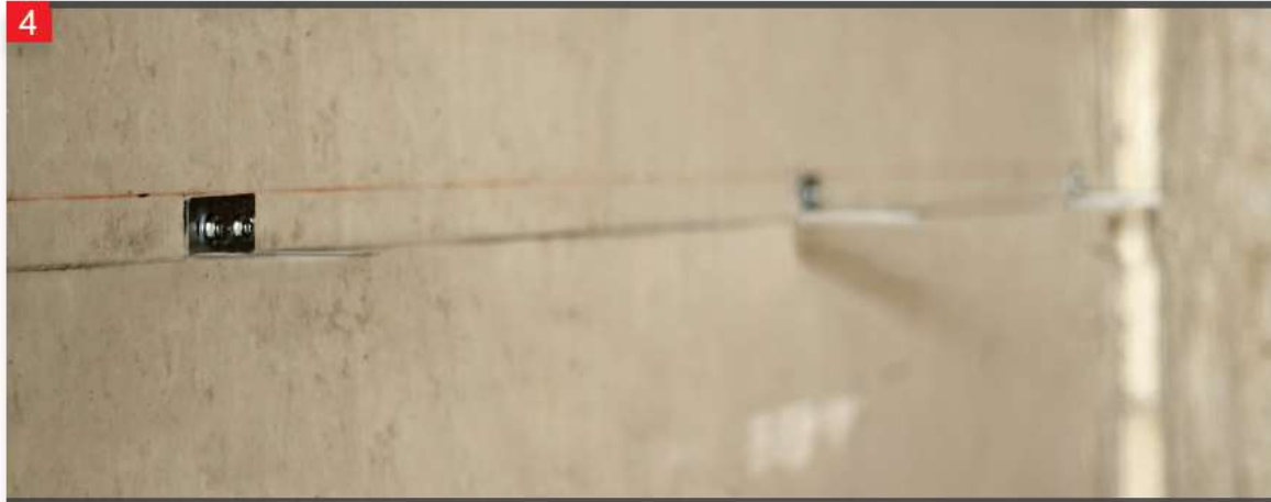
The L consoles for which the dowel locations have been marked are fixed into place using the right type of dowel.
