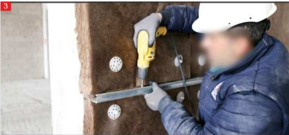
After fixing the stone wool on the wall surface the L profiles are attached to the L console with triphone bolts.
