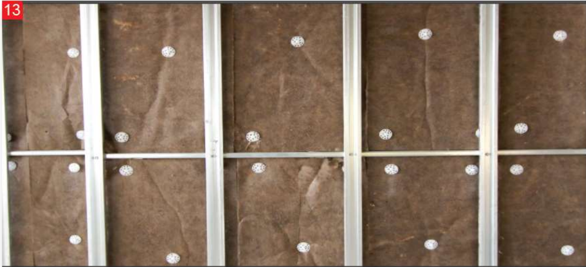
After the base construction stages are completed the panels are cut to the dimensions needed when starting the installation of the product.
