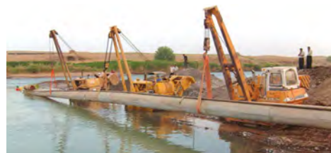
NATURAL GAS PIPELINE KHORMOR - ERBIL / N.IRAQ
