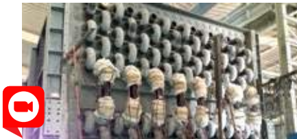
COILS and PIPING 30 - 37
