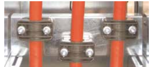
Adjustable cable supports
