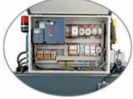
Elektrik Panosu Electrical Cabinet
