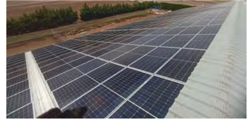
MESA SÜT / 518kWp / TEKİRDAĞ / 2018
