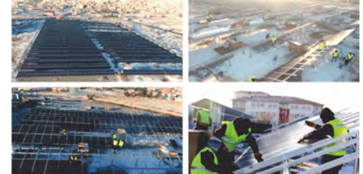
TALAS BELEDİYESİ / 1.15MWp / KAYSERİ / 2016
