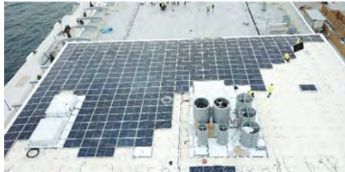
GALATAPORT / 150kWp / İSTANBUL / 2021
