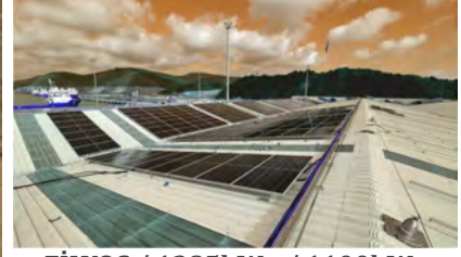
FİLYOS / 1385kWp / 1100kWe
