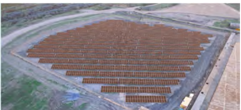
BAĞYURDU OSB GES / 1660kWp / 1600kWe İZMİR / 2023
